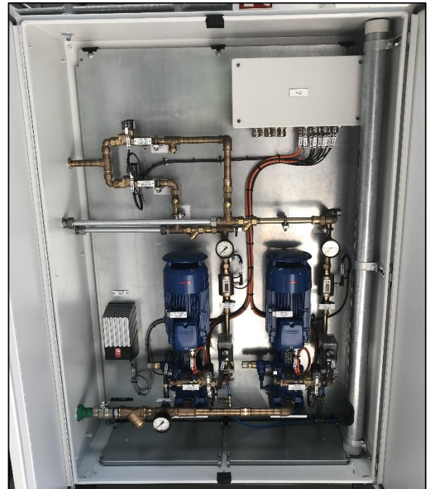
Wasserschrank Water cabinet
